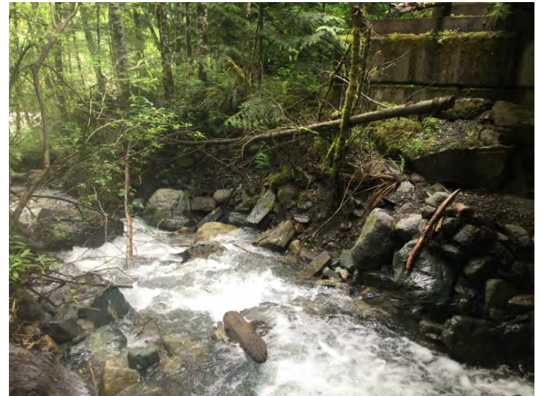
Downstream right bank riprap erosion
