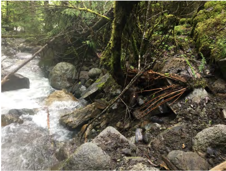
Downstream right bank riprap erosion
