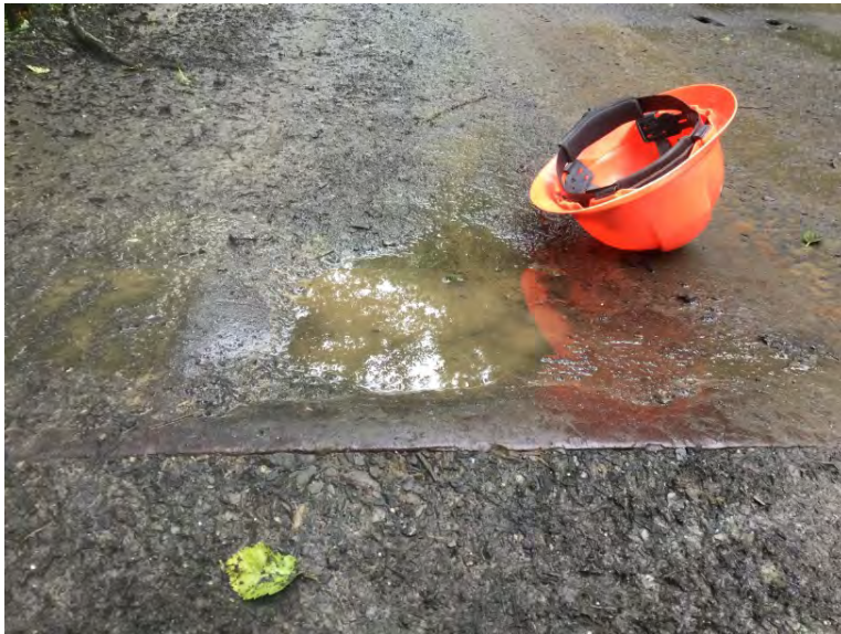
Running surface deformation on wheel path
